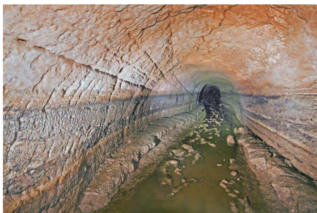
Surprisingly the canal tunnel isn't perfectly straight and has some wider sections. Note the historic water level marks - not much headroom!
